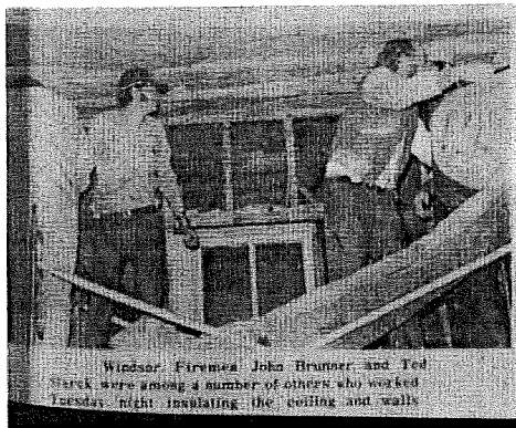
Fireman John Brunner and Ted Starck were helping install the ceiling and walls in the Depot
