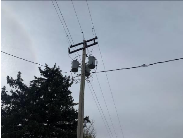
13. View of pole-mounted transformers located at the southwest site boundary
