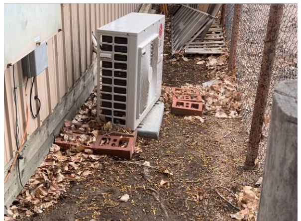
6. View of pad-mounted HVAC unit to the south of Pride Mechanical
