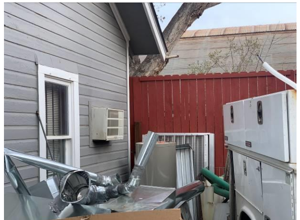
4. View of wall-mounted HVAC unit on the east side of the Post Office
